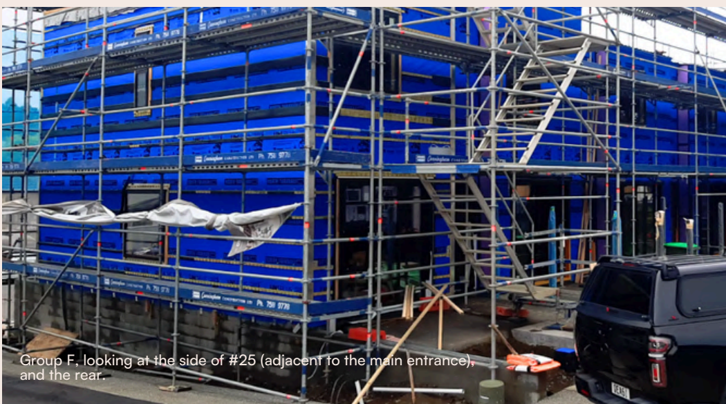
The frontage of Group F, commanding the site presence on the corner of Liardet & Pendarves Streets. Scaffolding up for cladding and glazing detailing.
