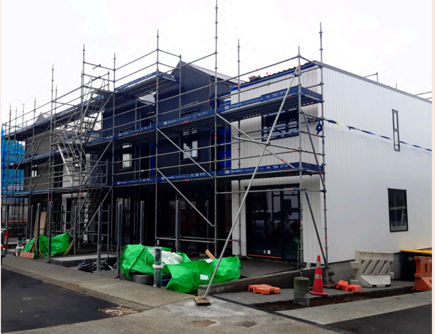
Exterior of Group G, from the rear, before courtyard fencing is installed.
