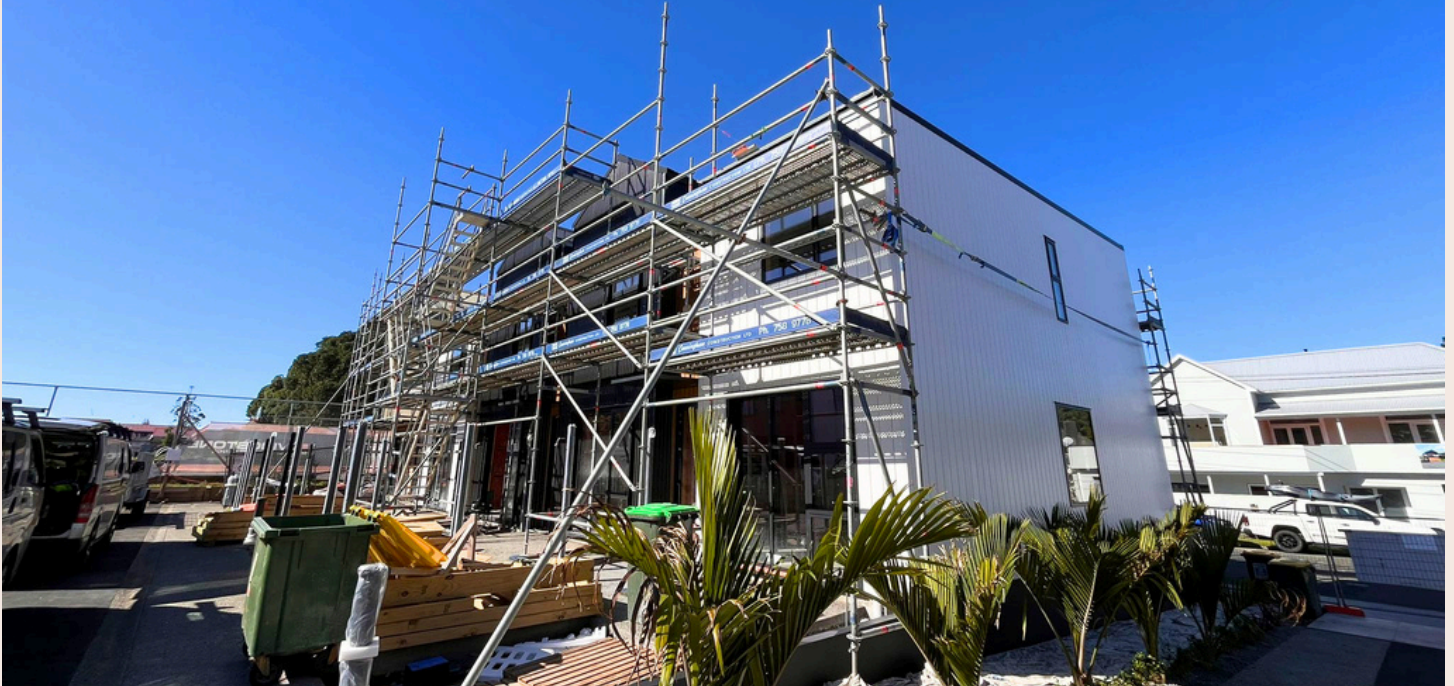
Exterior, Stage 3, Group G homes. Main entrance planting going in, with scaffolding up for the final exterior detailing.
